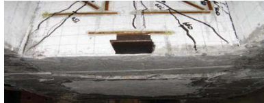
Fig. 6 Punching failure of joint section
